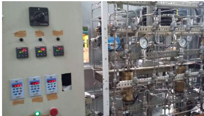
Figure 3-8. Electrocoalescence pilot plant
