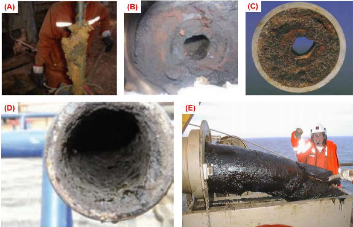
Figure 1 - The consequences of continuous wax deposition on (A) well tubing string, (B, C, and D) cross-section of flow lines, and (E) a pipe from a Norwegian production platform (extracted from Tukenov [9], with permission).
